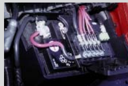
Figure 16: Bussed electrical center on the VW 1.8 turbo permits fewer splices and many separate current feeds, reducing the possibility of electrical glitches in the system.
